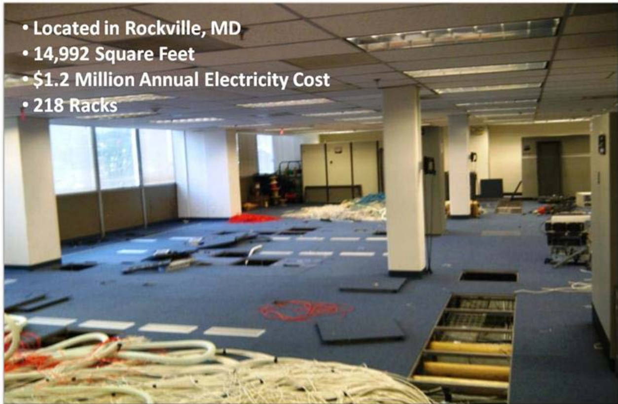
Figure 1: HHS Data Center, Shutdown Underway
